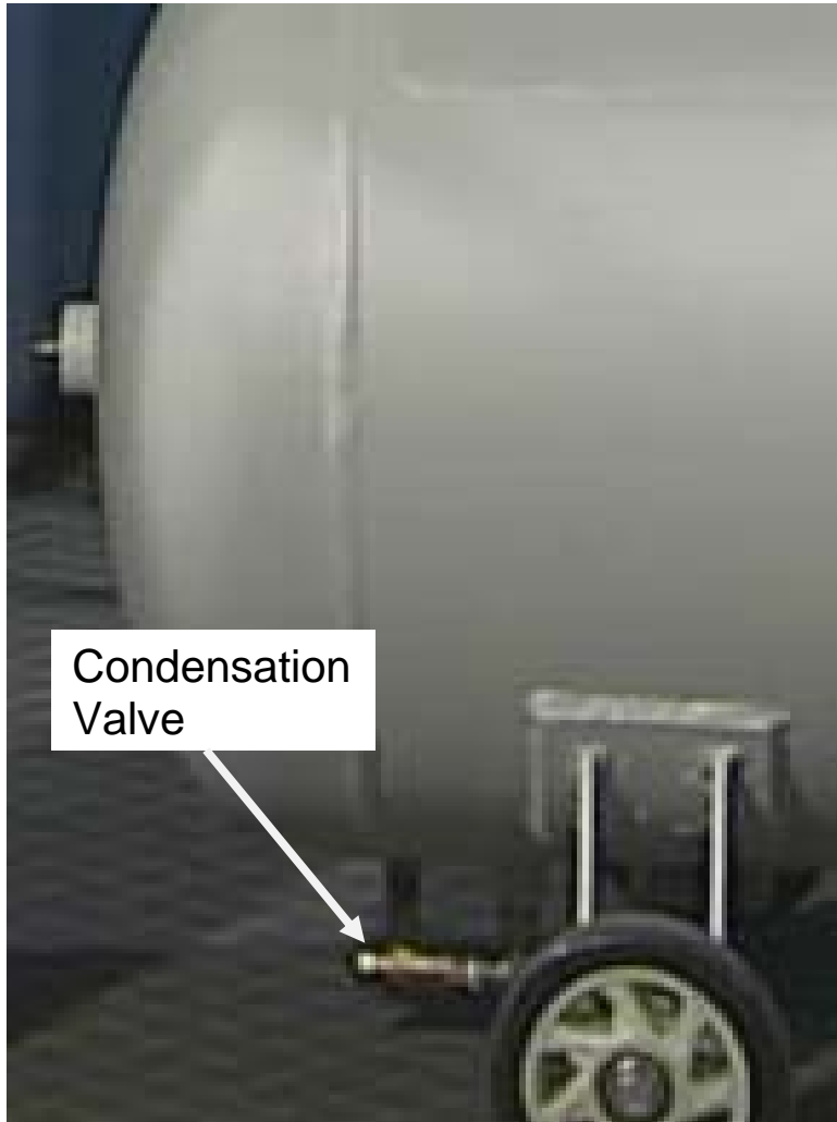
Condensation Valve Below Air Receiver Tank
